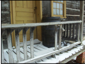
Broken railing on the Porch
